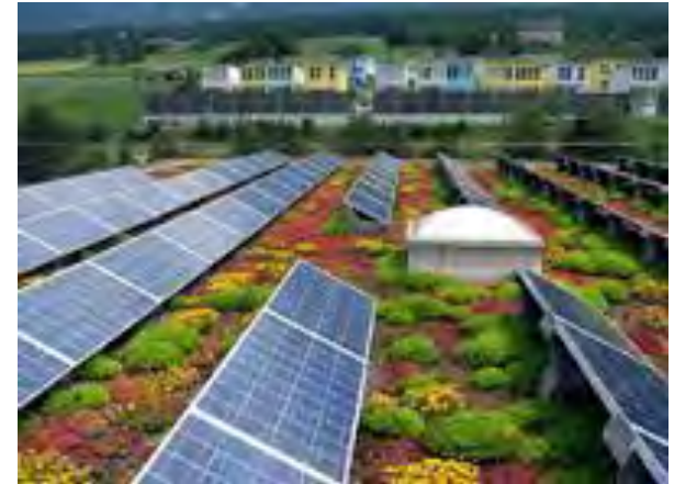
ROOFTOP SOLAR COLLECTORS
